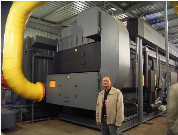
Me and the Broad - chiller.
