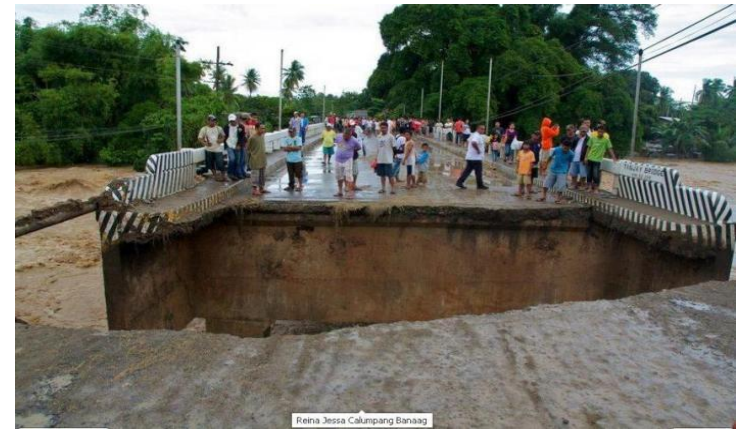
View from the eroded side of the bridge
