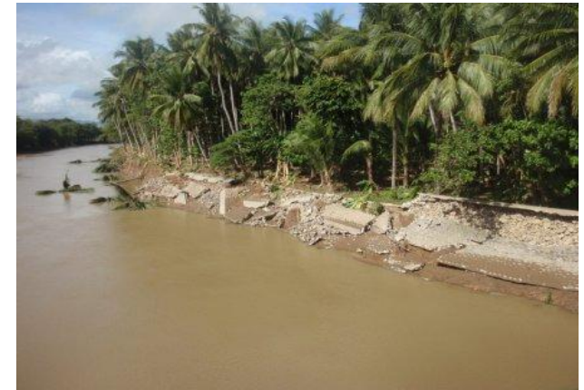
Up stream view of damage, Tabuc side
