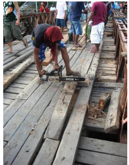
The lone chain saw on hand after it's repair. The chain had jumped off and the operator had to borrow tools from a nearby house.
