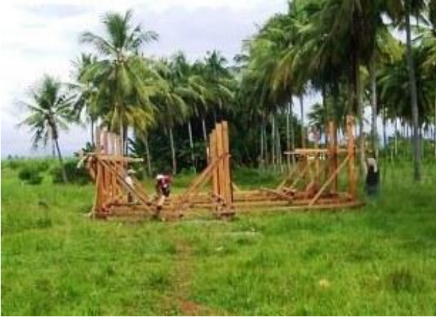
Day 4 of work by the master carpenter and his 2 helpers; posts are up, floor joists partly complete. They are on daily wage, not closed contract work.
